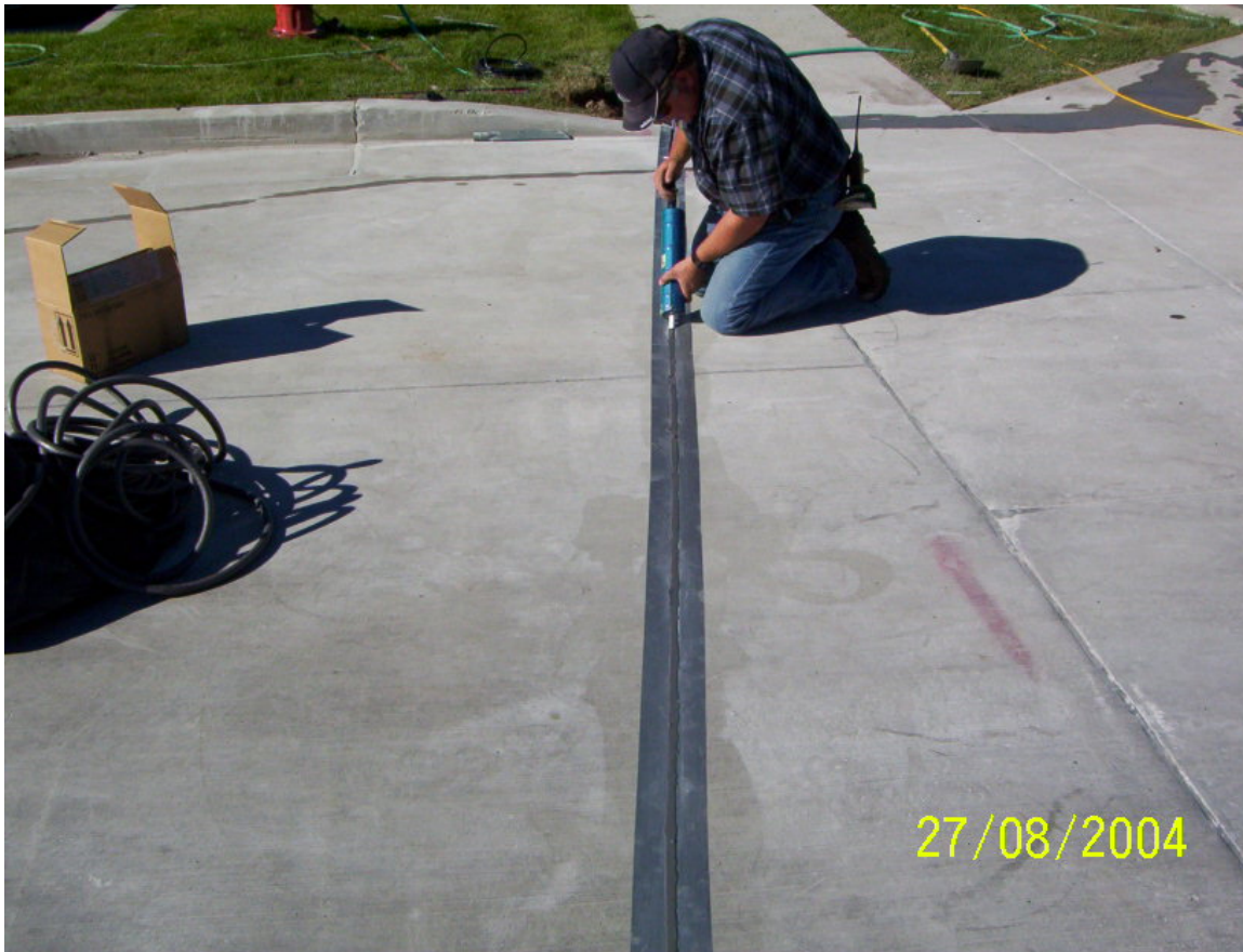
Figure 3-11. Application of the sensor cable epoxy. The saw cut is two inches deep. The backer rod is placed in the length of the saw cut below and above the sensor cable before epoxy application.
