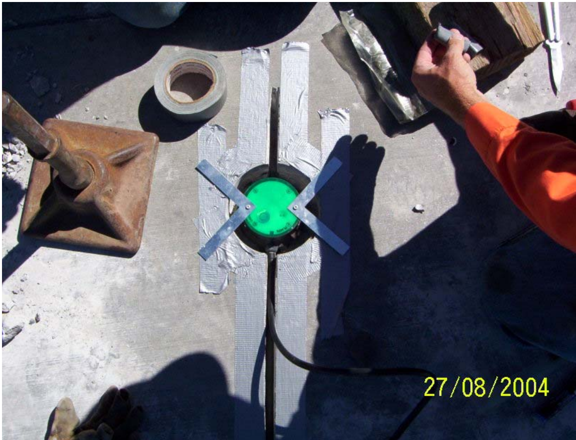
Figure 3-4. View of fast steel which is placed under the sensor prior to epoxy application to provide a base for the sensor.
